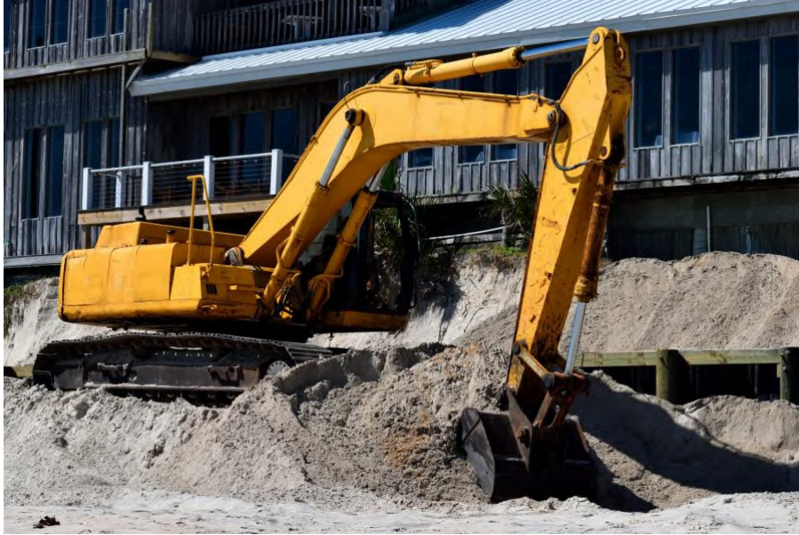
A backhoe working on beach erosion by Paul Brennan is released under a CC0 license
